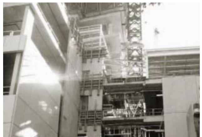
Melbourne's new County Court complex is the first Partnerships Victoria project. Building works are on target for the Court to be in operation during 2002.
